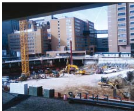
The construction site of the Genome Sequencing Center's new computer centre in St. Louis. Courtesy of Andras Horvath.
