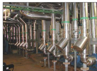
Dedicated pumps in the basement provide targeted air conditioning.
