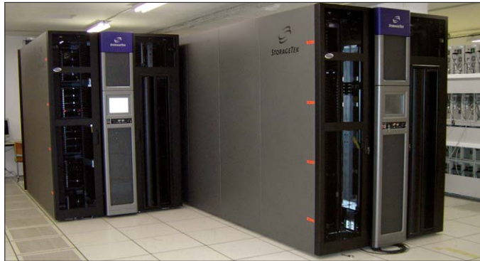
The Sun StorageTek SL8500 tape library in the Computer Centre.
