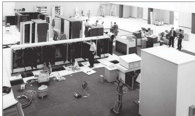
The computing centre was enlarged with the installation of a CDC 7600, which is shown here during its assembly in February 1972.
